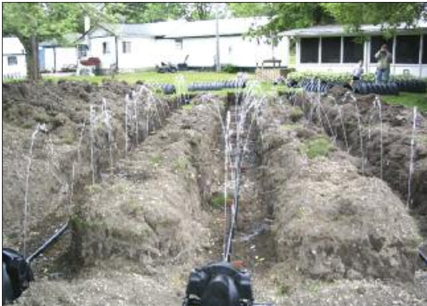
Shallow buried trenches showing equal distribution methods. Note: before placement of chambers.
